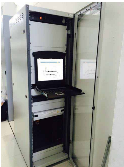
Fig. 8a: Server installation in a Control Room.
