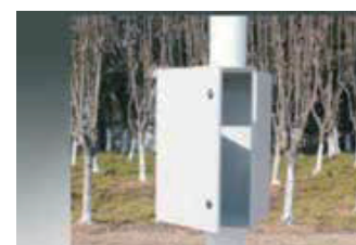
Fixed on the telegraph pole
